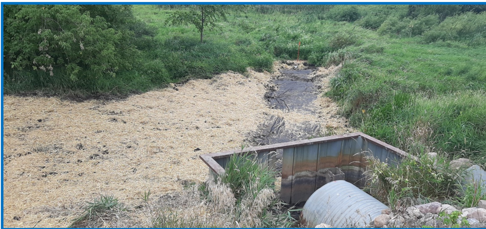
Clear Lake south side tributary iron-sand enhanced filter after maintenance in August, 2021
